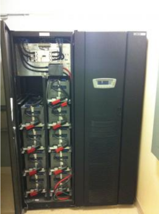
Uninterruptible Power Supply acts as the battery backup system for the facility
